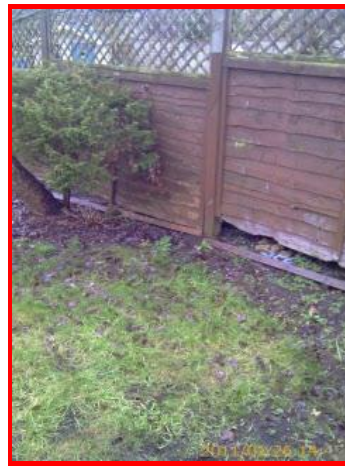
Fencing Boundary/Partition - damaged
