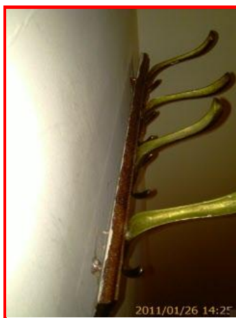
Coat Hook - loose
