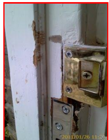
All Doors in Room Door frame - chipped
