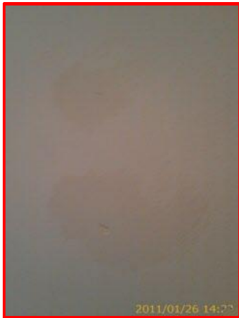
All Walls in Room Wall finish - over painted repair
