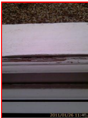
All Windows in Room Window frame/sill - chipped
