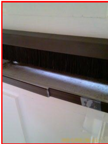
All Doors in Room Letter Box Cover - broken
