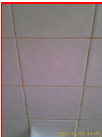
All Walls in Room Wall finish - dirty
