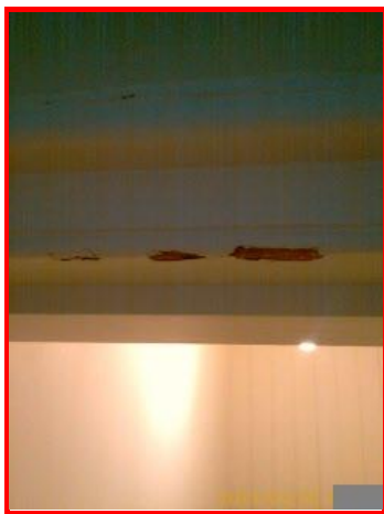
All Doors in Room Door frame - chipped
