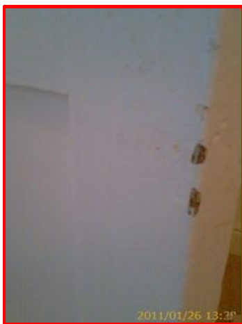
All Doors in Room Door finish - chipped
