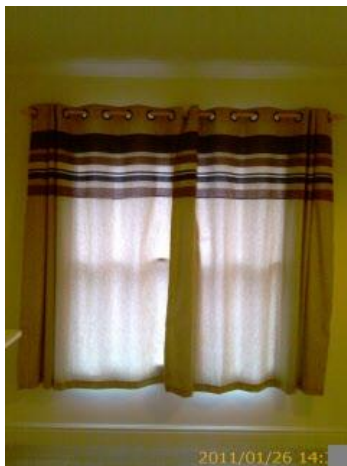
All Windows in Room All Windows in Room, Window frame/sill, Curtain Rail, Lined Curtains (below sill)
