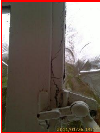
All Windows in Room Window frame/sill - chipped
