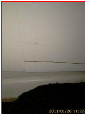
All Doors in Room Door finish - cracked (at bottom)
