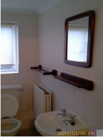
Toilet seat and lid, Toilet, Towel Rail, Radiator with cap, Sink, Sink plug, Taps - sink, Shelf, Mirror - wall
