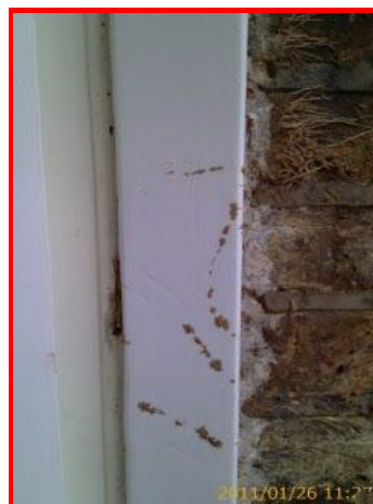
All Doors in Room Door frame - marked (in several places)
