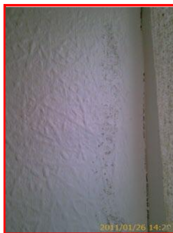
All Walls in Room Wall finish - black spot mould
