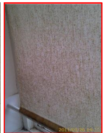
All Windows in Room Blind - black spot mould
