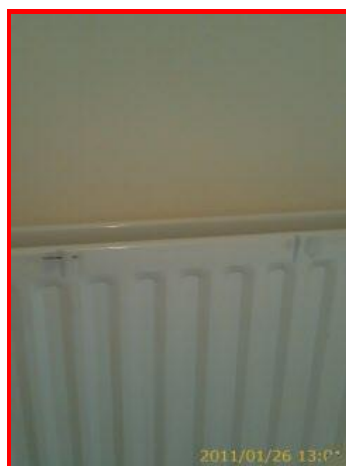
Radiator with no TRV or cap - marked
